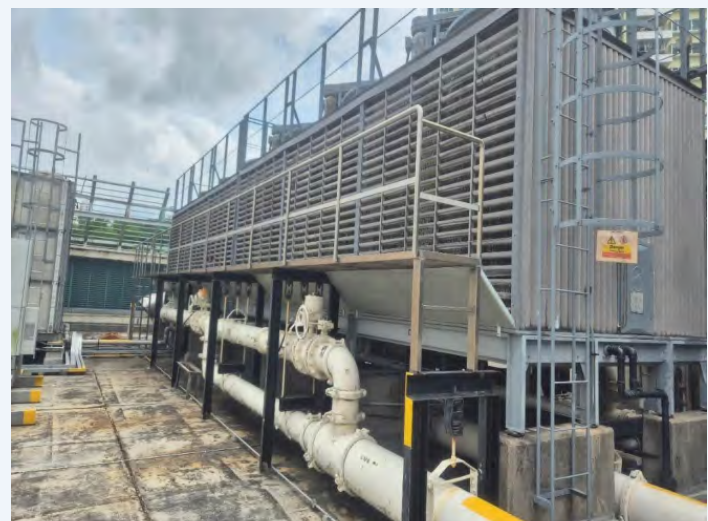
Figure 2: Provision of catwalk for safe, efficient, and effective cleaning of cooling tower fill media.
