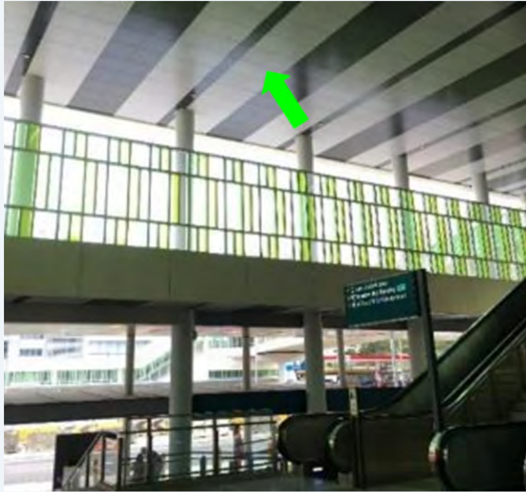
Figure 3: Moisture-resistant (e.g. aluminium), modularised ceiling panels are more durable and facilitate efficient maintenance since panels can be easily removed to access concealed services.
